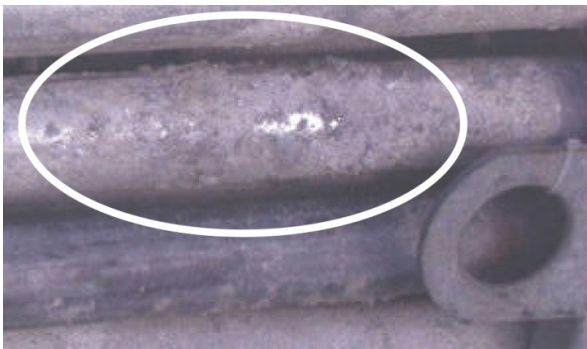
Photo 11 Impermissible large crusts of concrete
