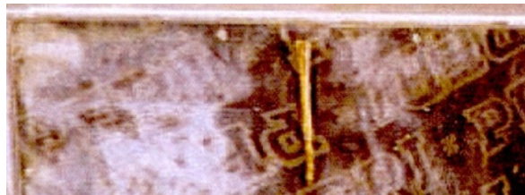
Photo 19 Impermissible scratches in the formlining (Depth > 1 mm)
