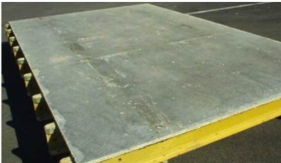
Photo 21 Permissible cleaning condition
