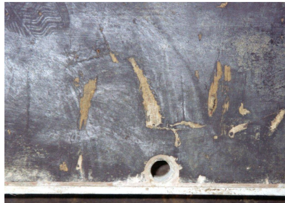
Photo 2 Impermissible damage in the formlining (depth greater than 1 mm, surface veneer penetrated)
