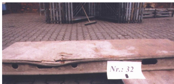
Photo 20 Impermissible damage on the frame profile
